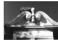
Features such as window hoods, brackets and columns are often associated with particular styles and therefore their preservation is important.
