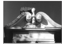
Features such as window hoods, brackets and columns are often associated with particular styles and therefore their preservation is important.
